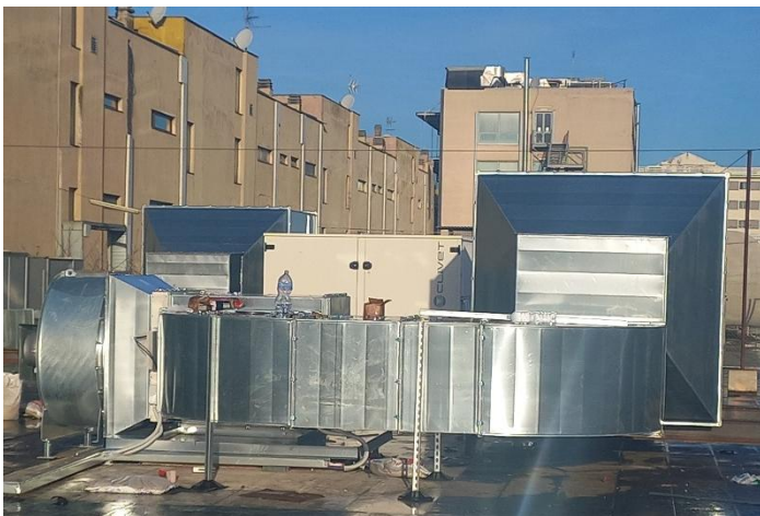
ROOF TOP & Smoke Extractor F400
